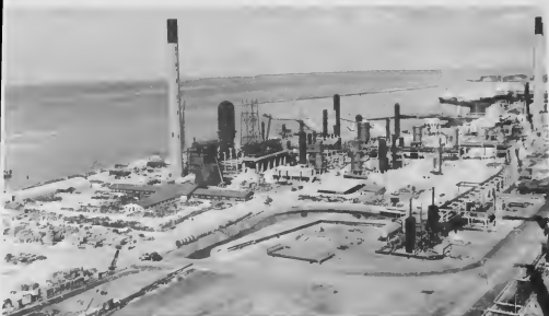
Work in progress on Oct. 1, 1970 on new Hydrodesulfurization units on reclaimed area.
